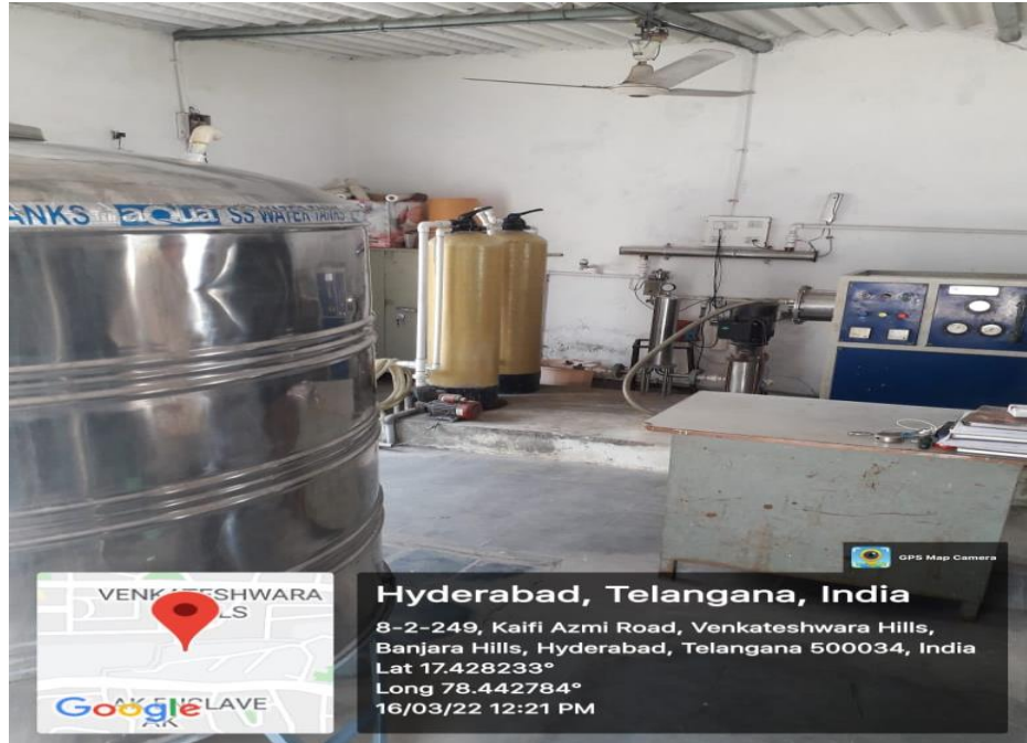
RO Plant-I Facility
