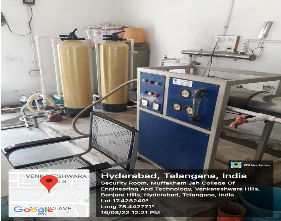
RO Plant-I Facility
