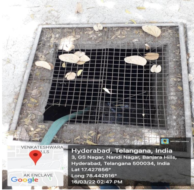
Waste Water Recycling Sump - I
