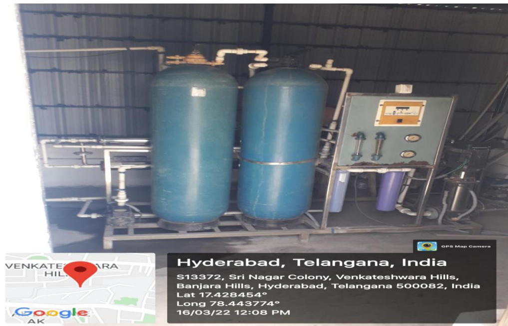
RO Plant-II Facility
